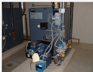
One of the boilers servicing the building
