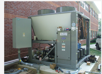
New Carrier High-Efficiency Chiller
